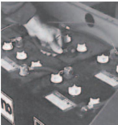
6-Check battery terminals
